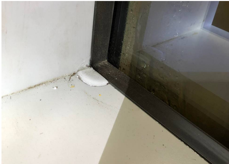
Photo 1: Water observed during test 10
